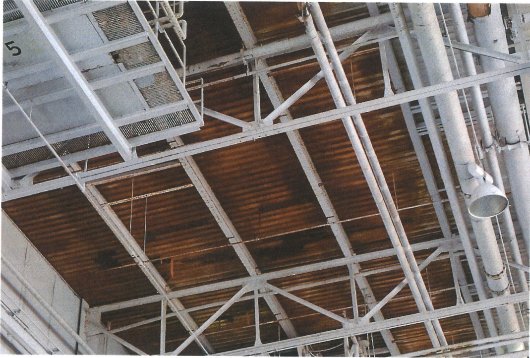
Closer look at corrosion
