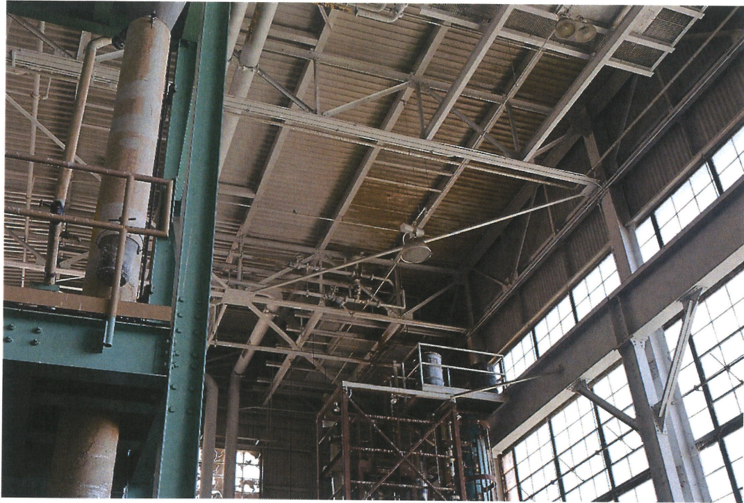
Corrosion on Northeast side of roof between columns EF13/EF14 and F13/F14
