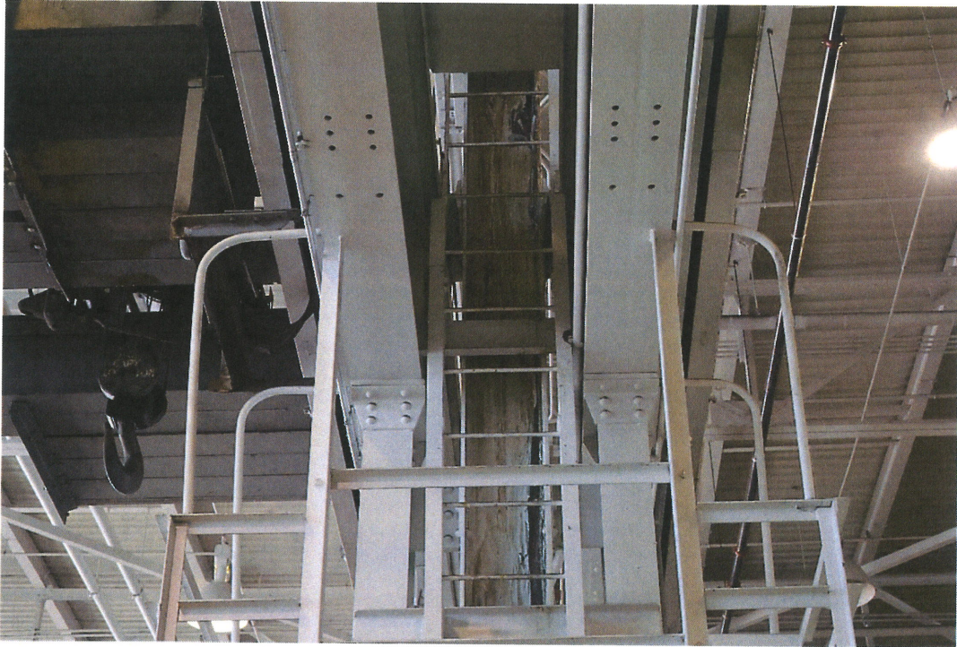
Evidence of water leak on column B3
