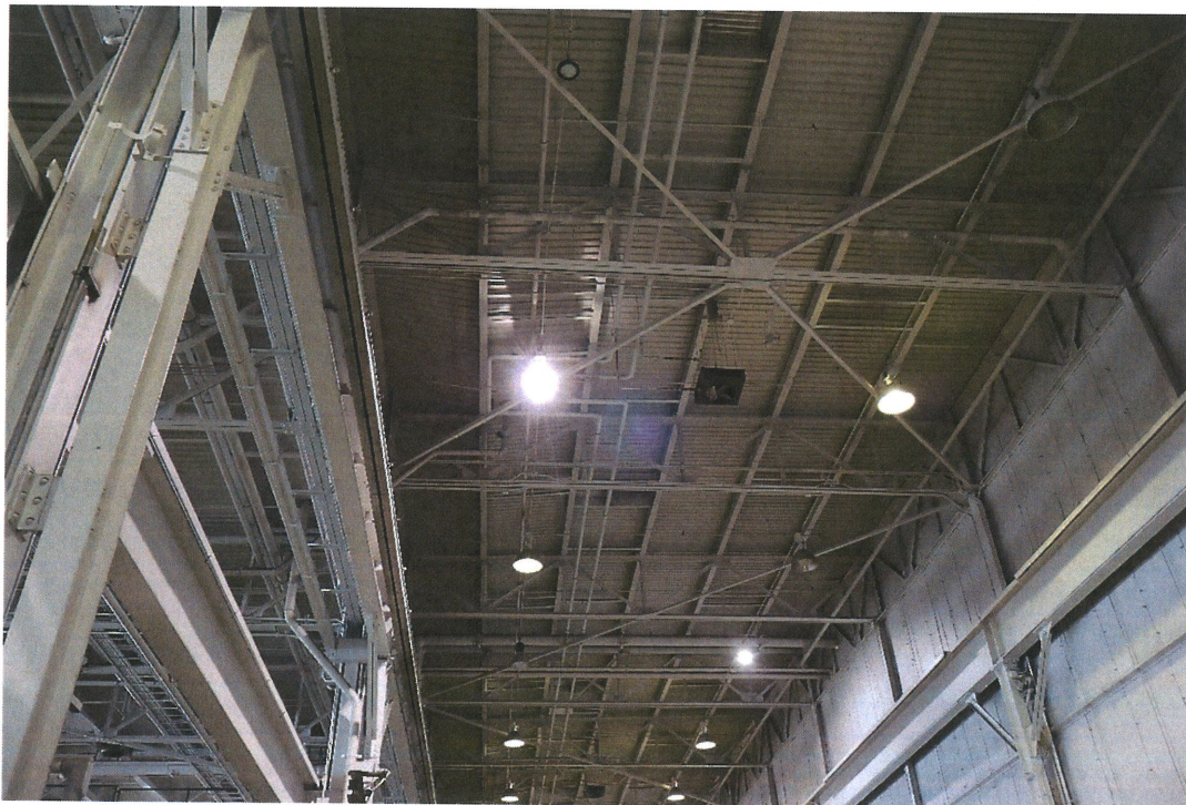
Looking North in Highbay
