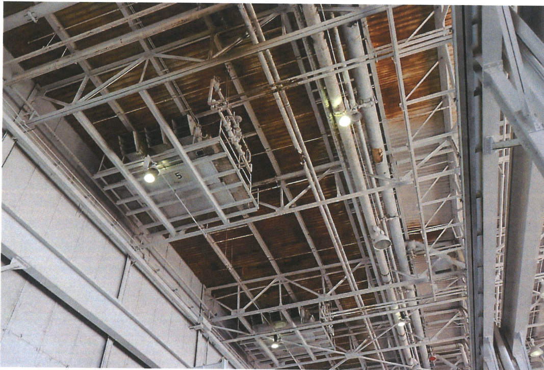
Corrosion in large area of roof between columns D4/D7 and E4/E7
